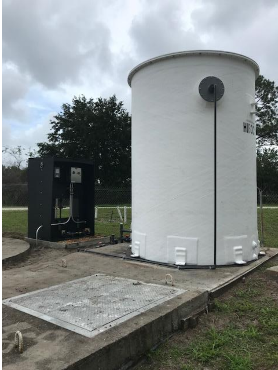
HIBOCS 200 – Installed at Brevard County (Tucker Lane Lift Station)
